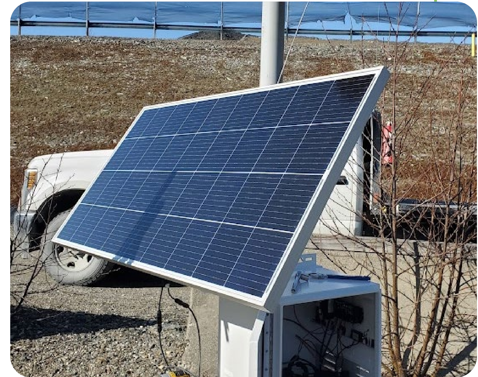
Installation of solar powered dust monitor at Greens Creek mine tailings facility
