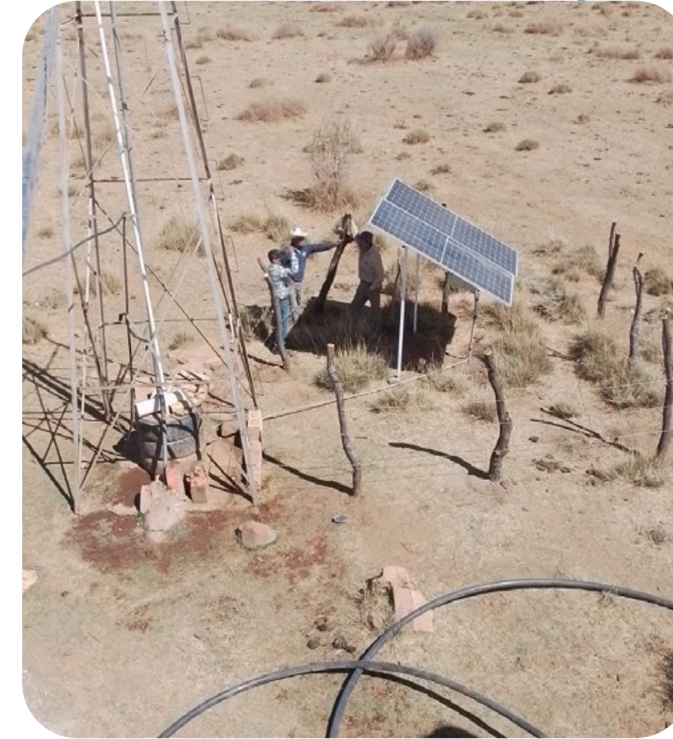
Solar powered pump at San Sebastian
